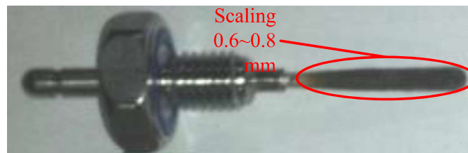
Figure 10. Deposit on grading electrodes at anode side of valve assembly of rectifier station
