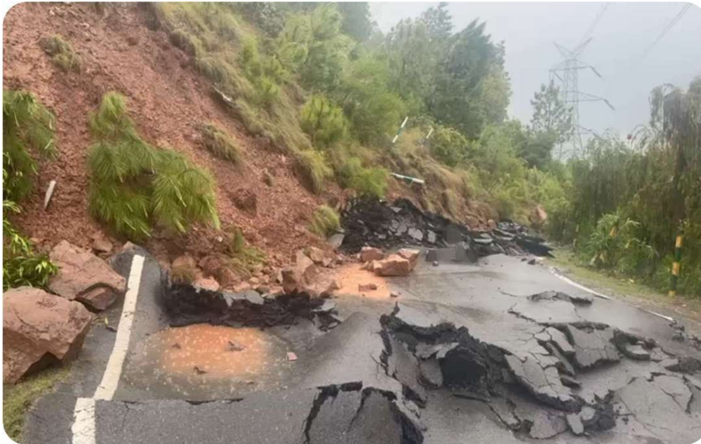
Damaged connecting road
